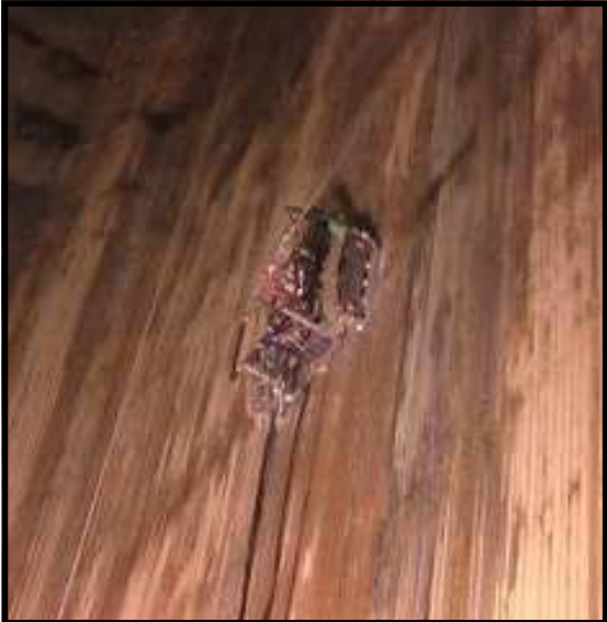
Tube wall thickness inspection (UT, line scan), TVA Kingston Unit 9, approx. 5 mins per tube (100' length), 10 hrs per wall
