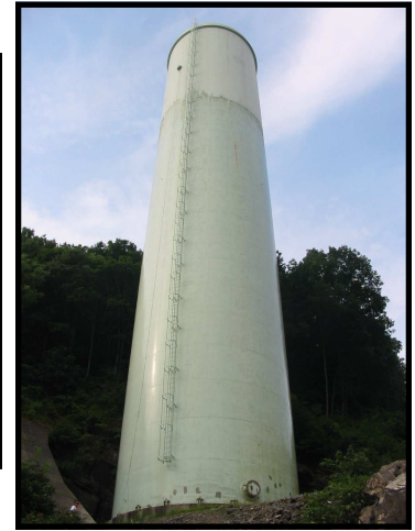
NDE inspection, TVA South Holston Dam Surge Tank, 12 vertical passes, thickness measurement every 6 inches, total inspection time 4 hrs. including setup
